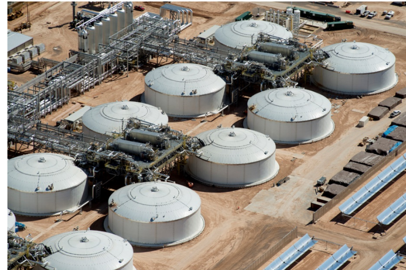
Source: Solana CSP plant (US), Caldwell Tanks
